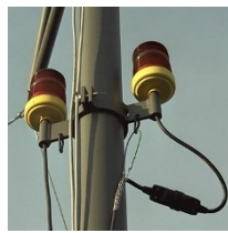
Night warning beacon
